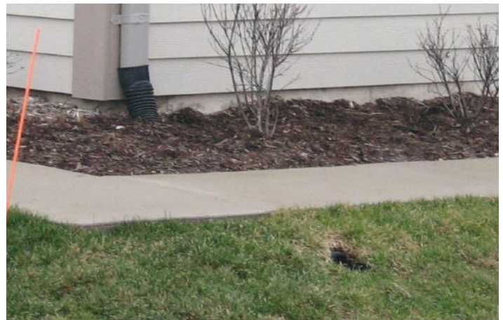
The drain slopes away from the foundation and terminates at the proper distance
