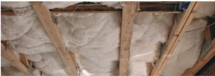
Insulation has misalignments, compression, and gaps.
